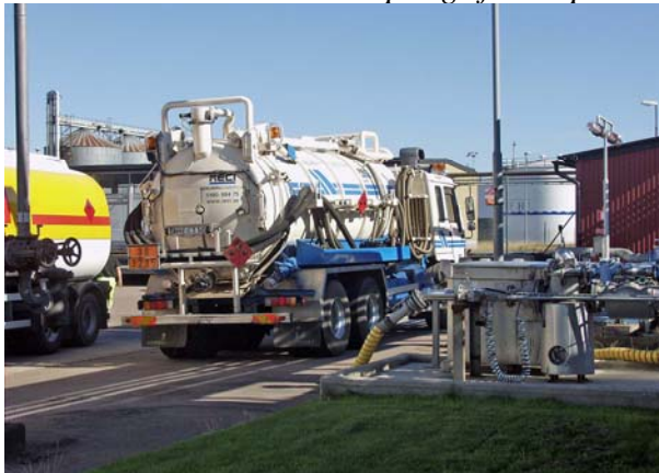
Picture 7: Sludge reception facilities
